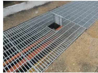
Steel grating trench covers
