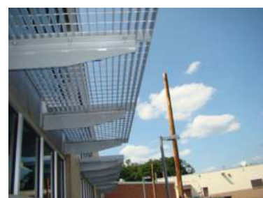
Steel grating sun shade panels
