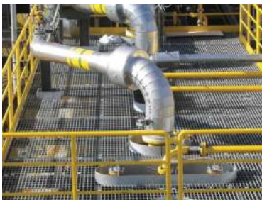
Steel grating platform
