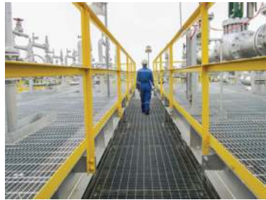
Steel grating platform walkways
